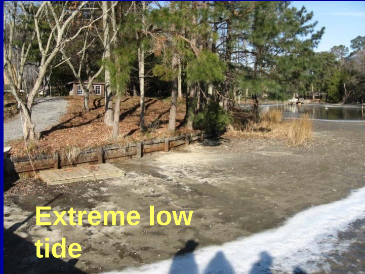
Before – failing timber bulkhead
