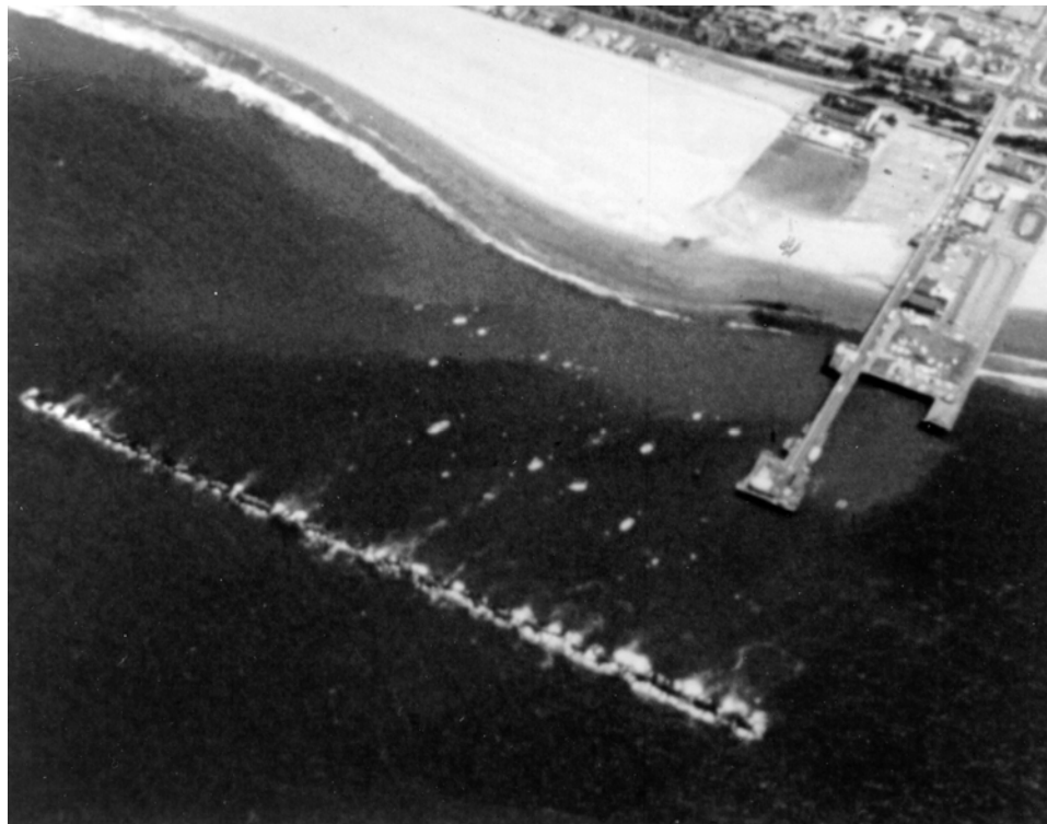
b. Deteriorated breakwater allowing wave transmission
