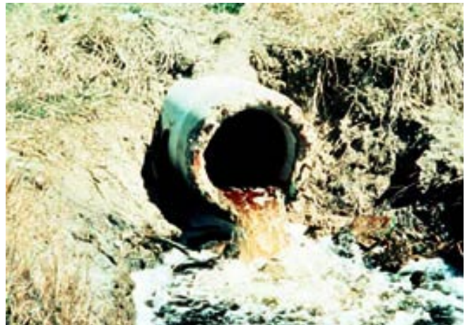
Figure 13. Contaminated outfall; point source pollution.
