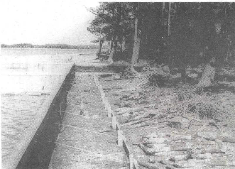
The proper design and construction of a bulkhead include the use of tiebacks and filter cloth.
